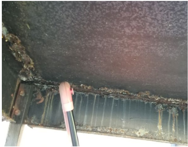
Photograph 10: Oxidization underneath exterior stairwell
