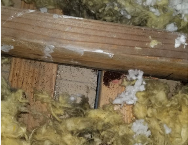
Photograph 13: Unit 201. Termites infestation
