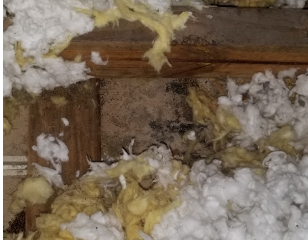
Photograph 14: Unit 203. Termites infestation
