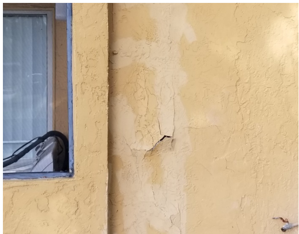
Photograph 12: Exterior wall cracking
