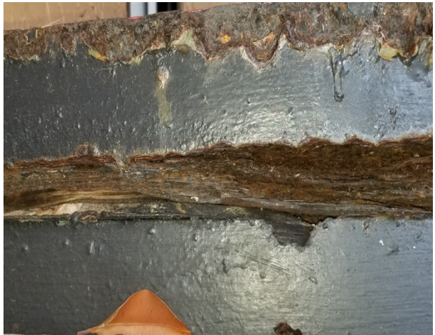
Photograph 10: Unit 202. Oxidization on stairwell
