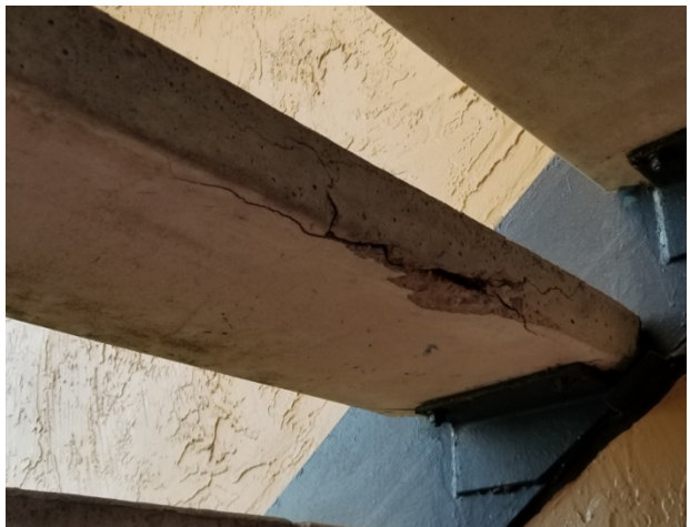
Photograph 12: Cracks on the stairwell steps
