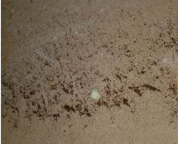
Photograph 13: Unit 203. Termite infestation
