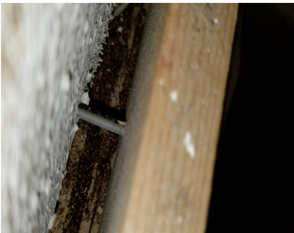
Photograph 11: Unit 201. Termites infestation
