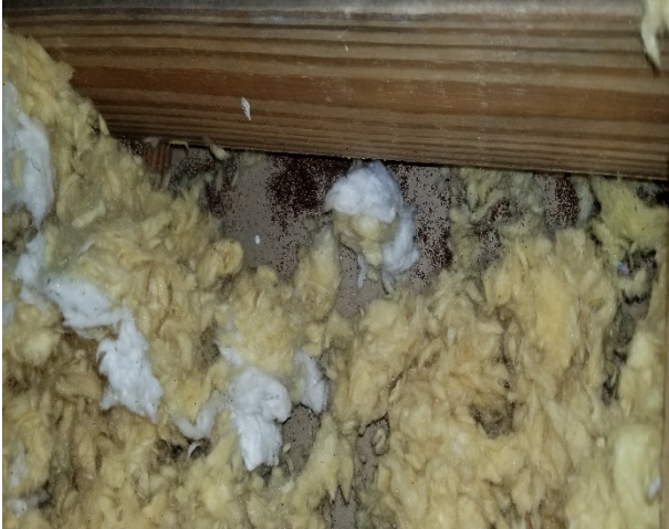
Photograph 13: Unit 205. Termites infestation
