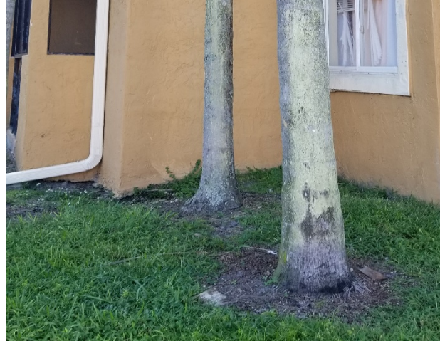
Photograph 14: Tree roots growing against the foundation
