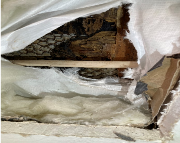
Photograph 7: Unit 206. Deteriorated sheathing
