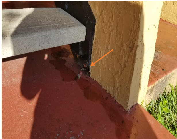
Photograph 16: Corroded connection for the common metal staircase
