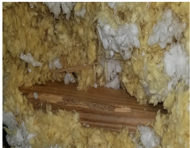
Photograph 12: Unit 203. Termites infestation
