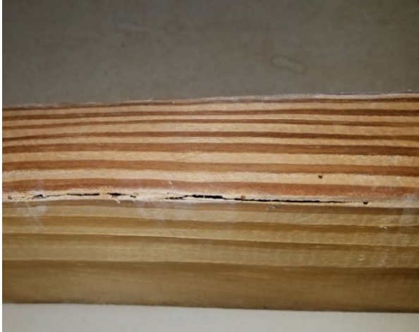
Photograph 7: Unit 205 cracked wood joists within attic
