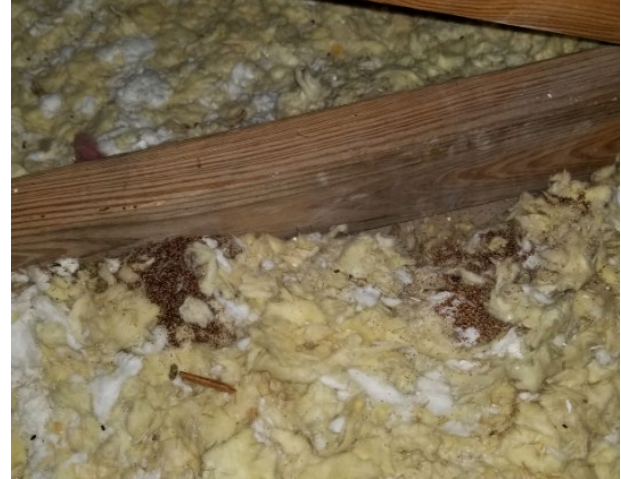
Photograph 14: Unit 208. Termites infestation
