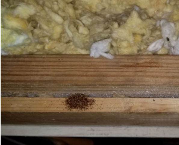
Photograph 13: Unit 202. Termites infestation
