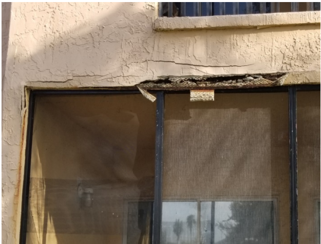
Photograph 12: Exterior wall cracking and exposed wire lath
