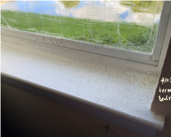
Photograph 3: Unit 103. Termites droppings
