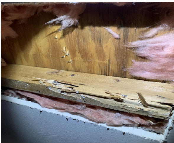
Photograph 11: Unit 205. Termites Damage
