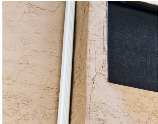
Photograph 10: Exterior wall cracking
