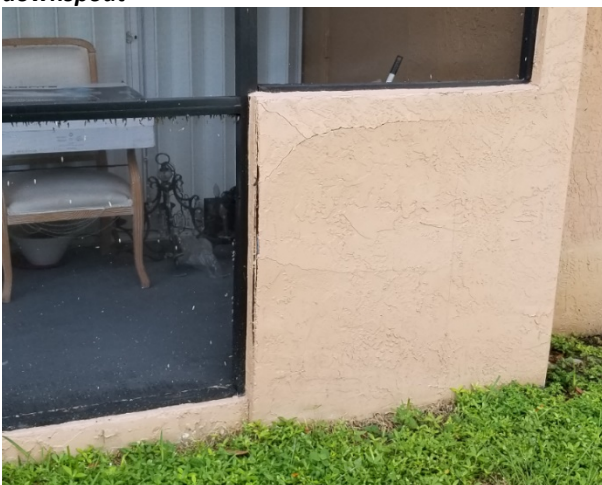
Photograph 11: Exterior wall cracking
