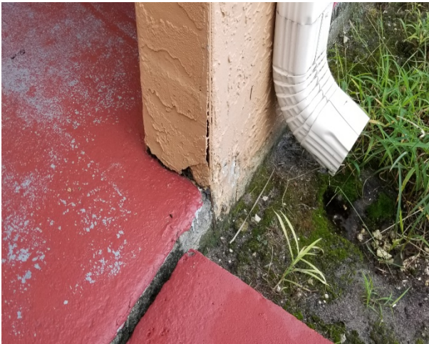
Photograph 9: Corner crack on exterior wall near downspout
