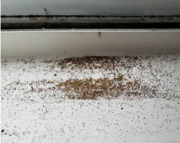
Photograph 13: Unit 208. Termites infestation
