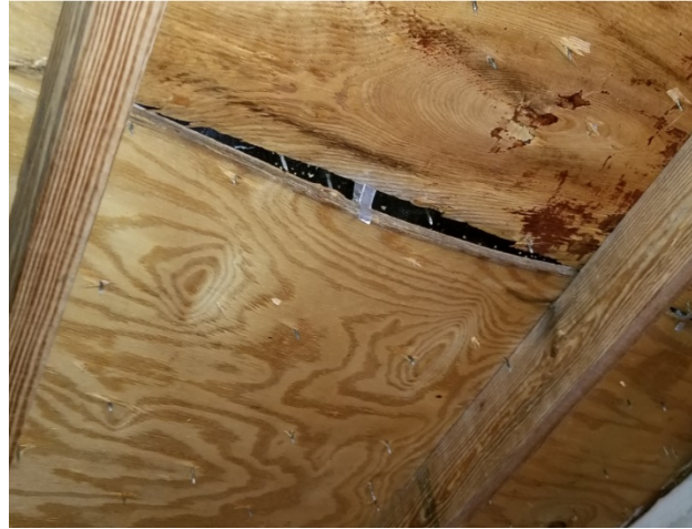
Photograph 14: Unit 208. Opening within the attic sheathing
