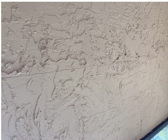
Photograph 11: Cracks on balcony ceiling Unit 104
