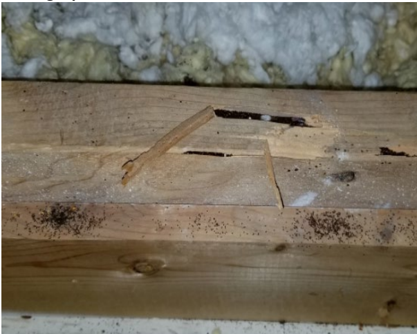
Photograph 5: Unit 202. Termite Infestation
