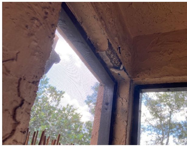
Photograph 12: Exposed wire lath on Unit 204 balcony
