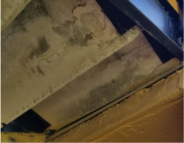
Photograph 13: Exterior staircase. Spalling and cracks
