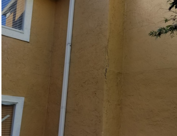
Photograph 14: Cracks on the exterior walls
