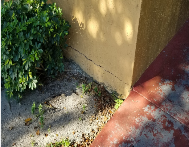
Photograph 13: Soild washout and exterior wall crack
