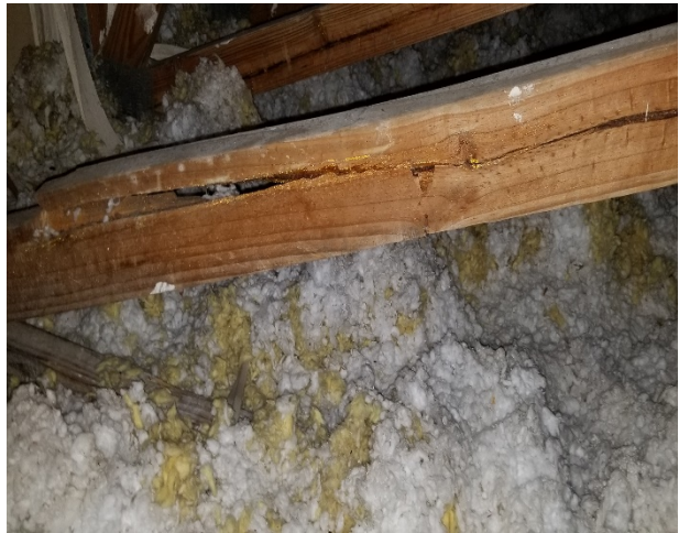
Photograph 10: Unit 202. Isolated damage to roof truss
