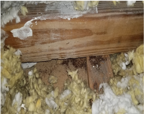
Photograph 9: Unit 201. Termite infestation
