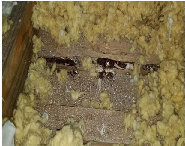
Photograph 12: Unit 208. Termite infestation
