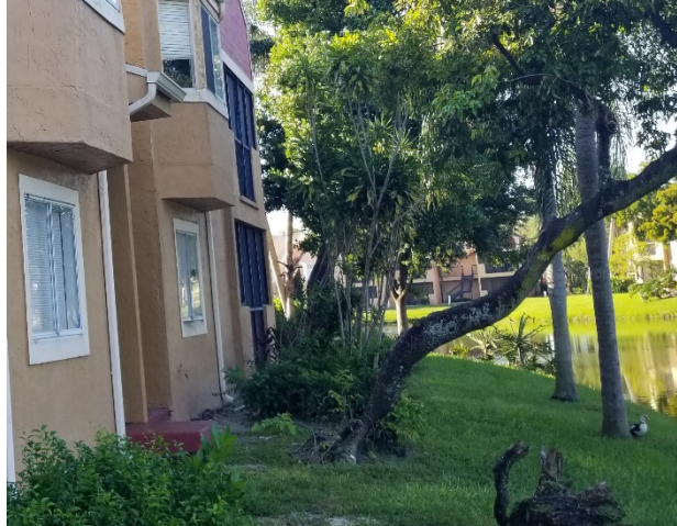
Photograph 14: Tree roots growing against the foundation
