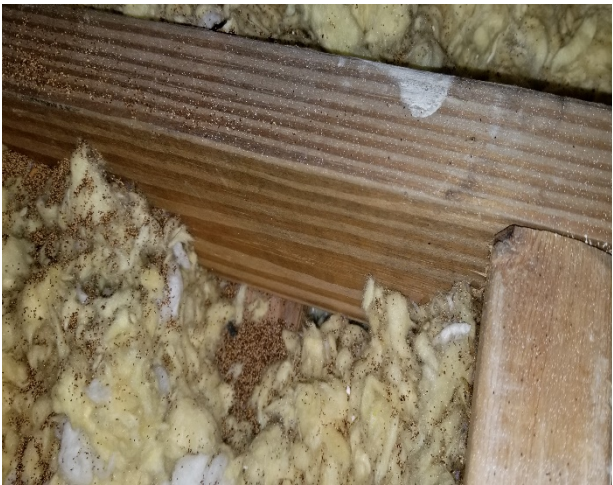
Photograph 11: Unit 207. Termite infestation
